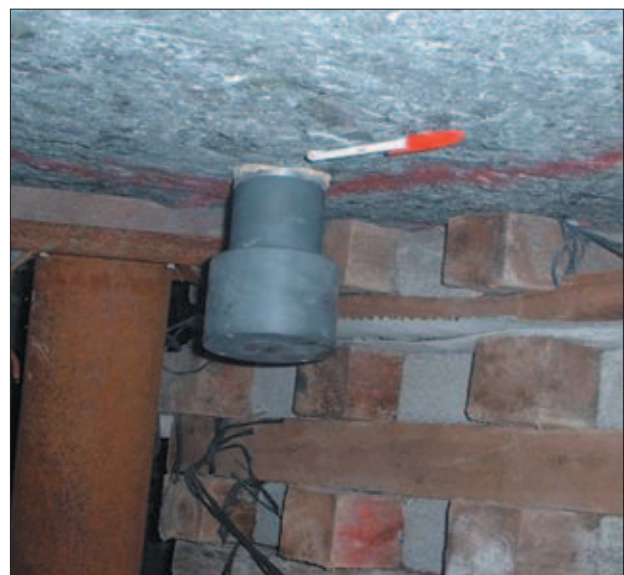
Figure 1—Underground installation of peak velocity detector
